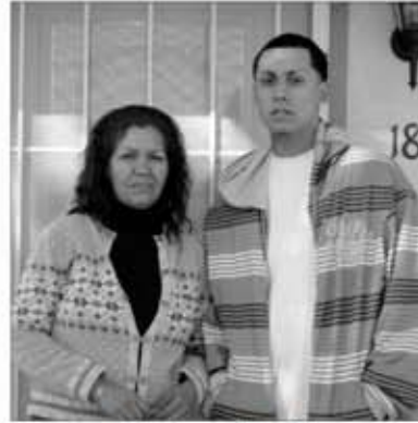
Enriquez Family Fund for Humanity and Federal Home Loan Bank Wish program (Renovation) Phoenix
